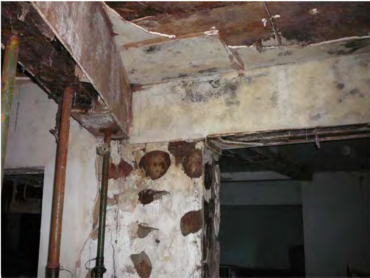
Photograph 13: Damp ingress to ground floor & corrosion to steel beams
