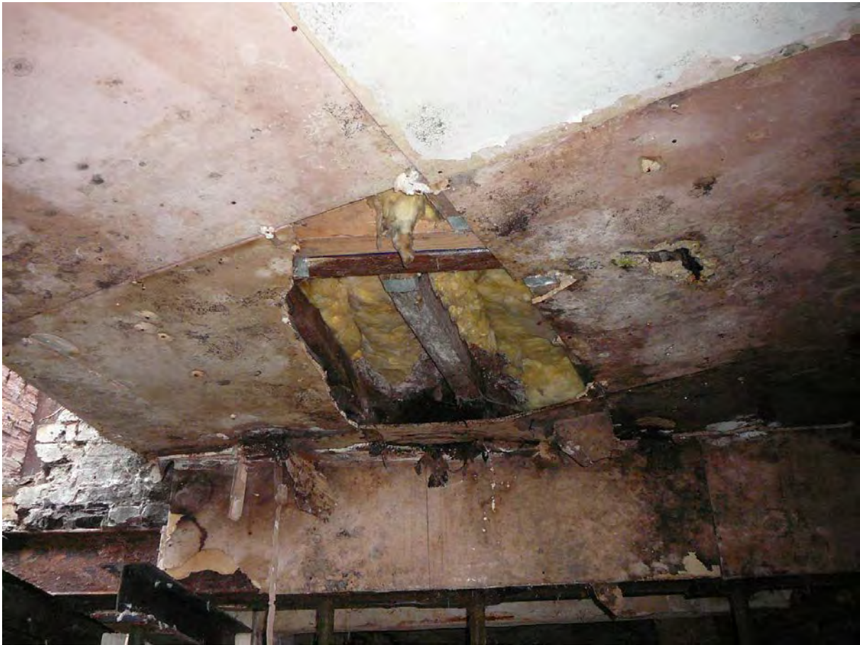
Photograph 5: Loss of ground floor ceiling and fire damage to first floor
