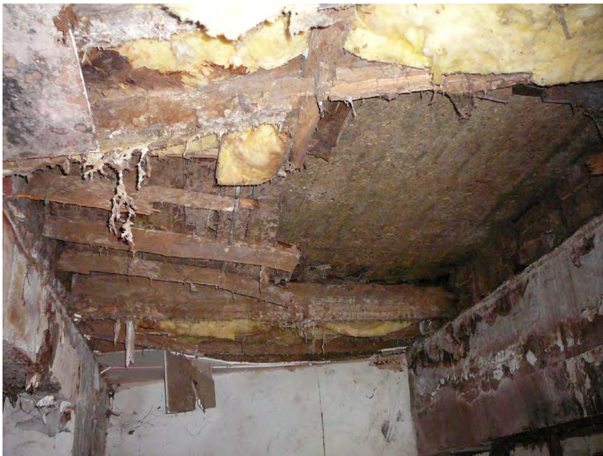
Photograph 9: Timber rot to first floor - 1
