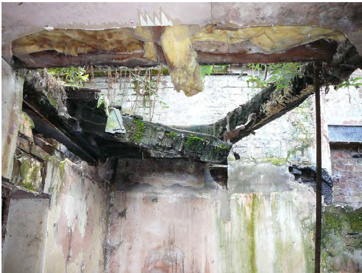
Photograph 7: Fire damaged first floor – 1
