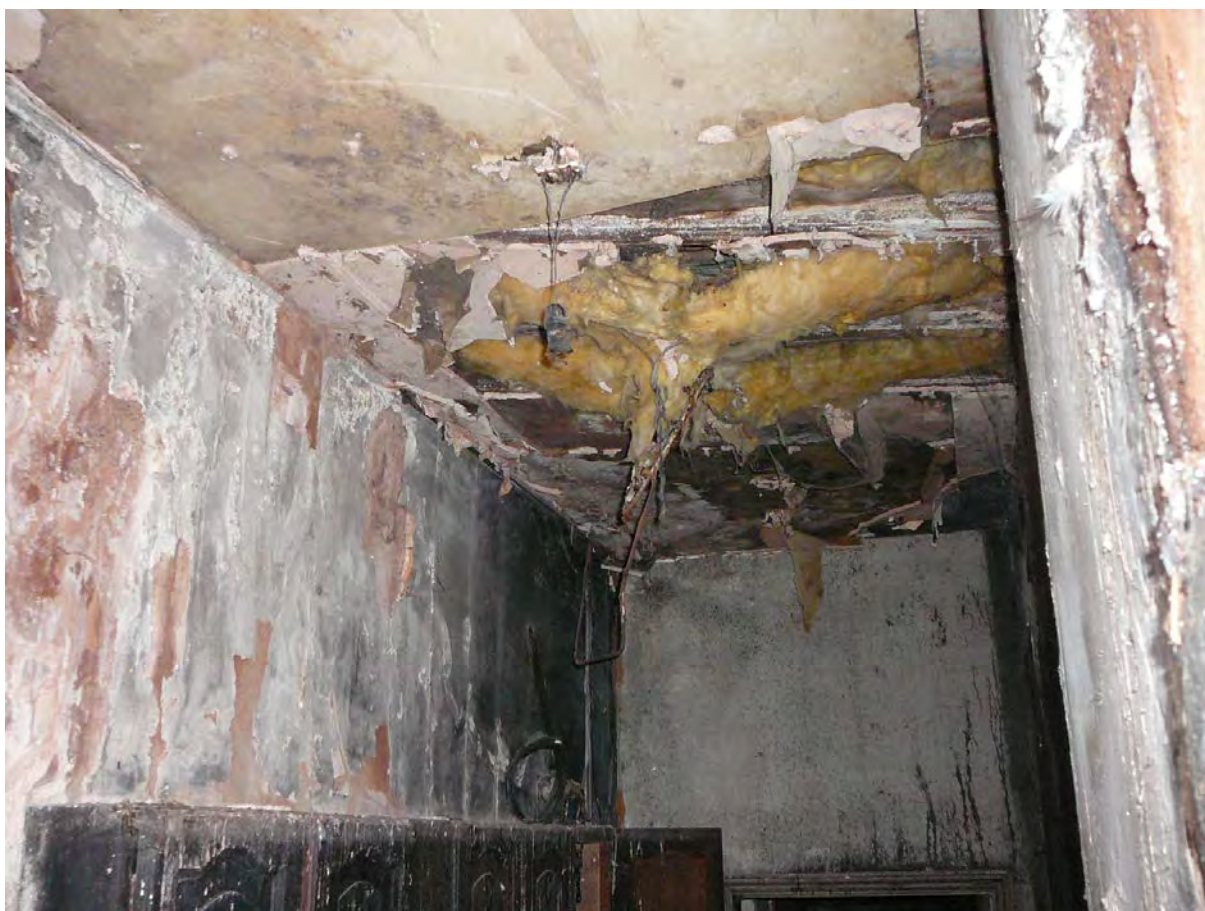
Photograph 8: Fire damaged first floor - 2
