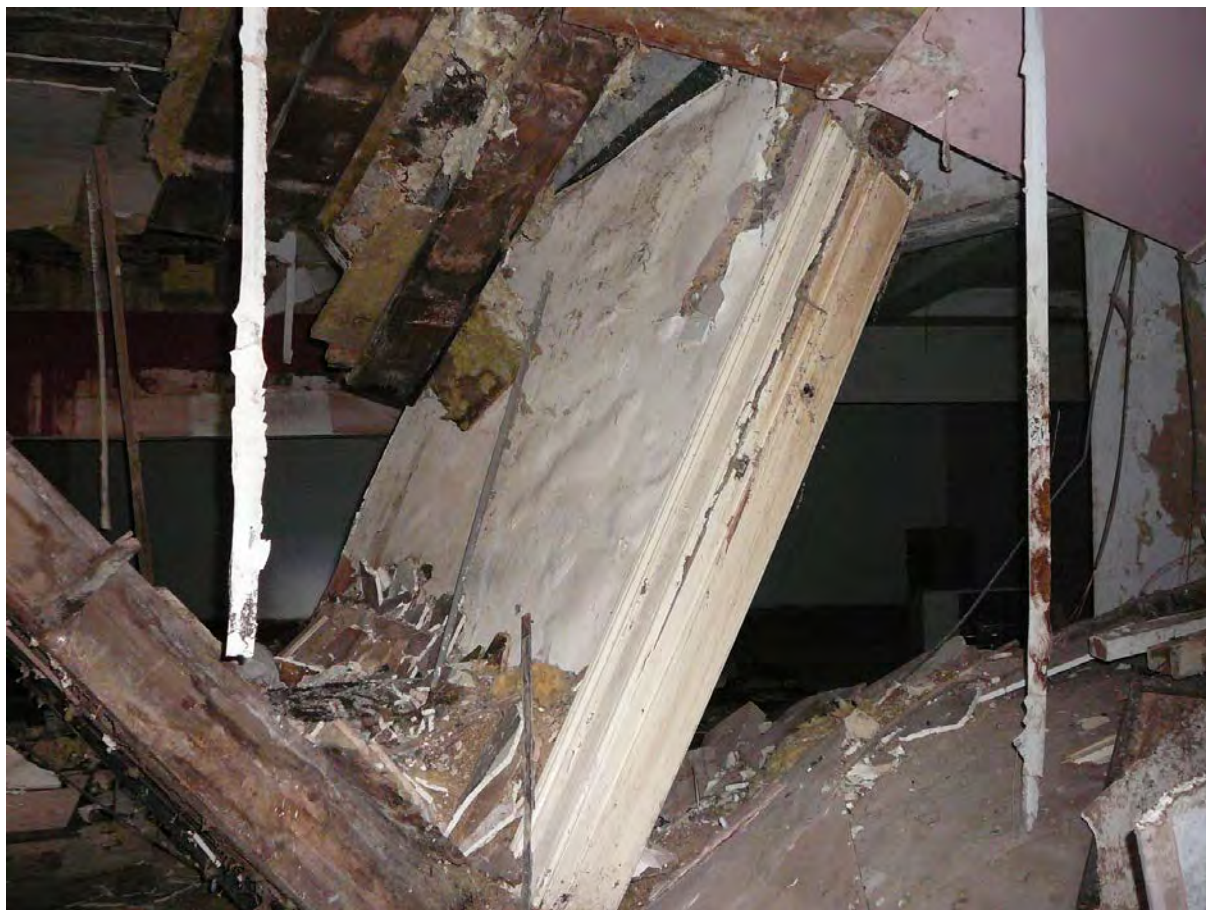
Photograph 11: Part of collapsed second floor
