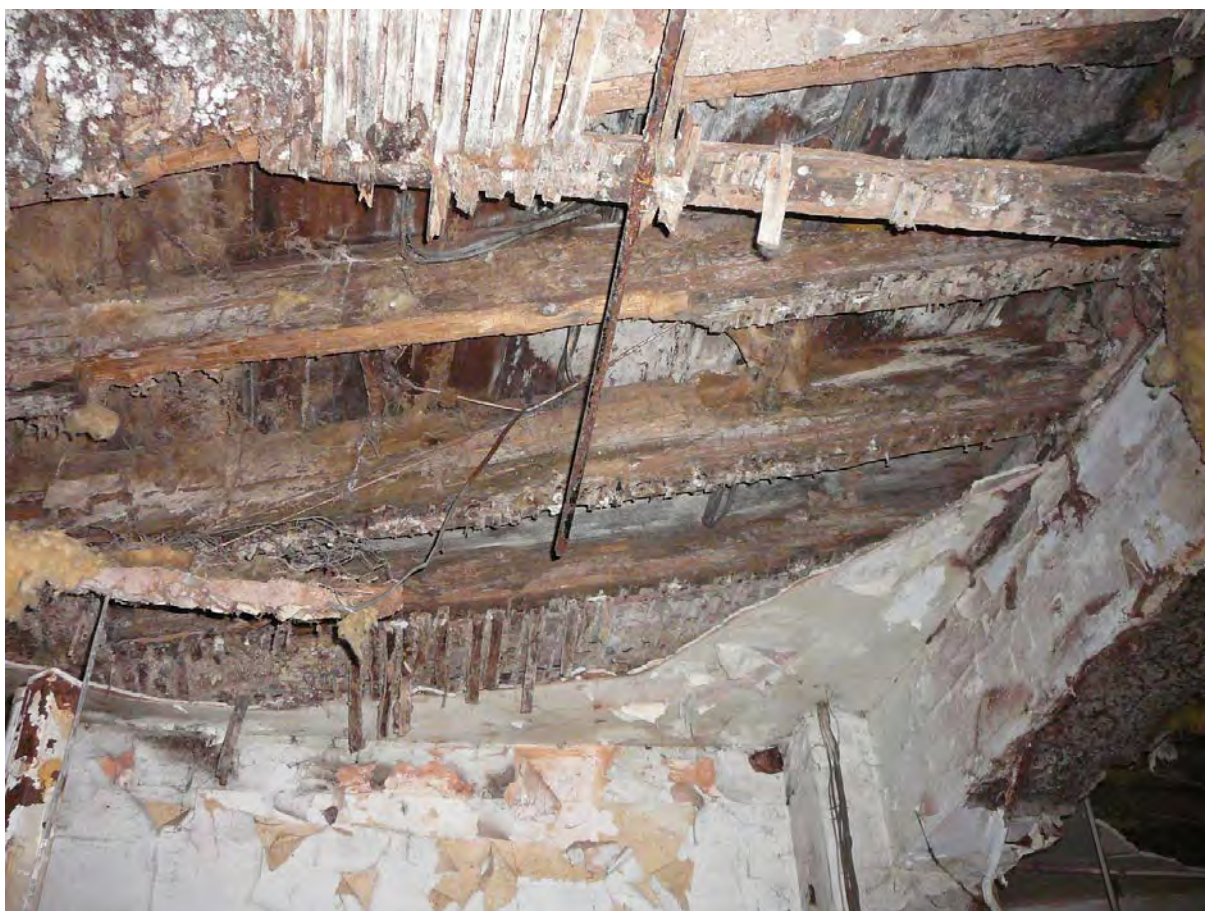
Photograph 10: Timber rot to first floor - 2
